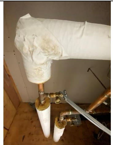
P2 Straight run fiberglass insulation
