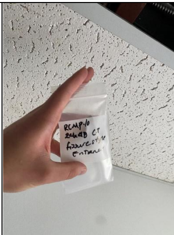
P1 – typical fissure design ceiling tiles
