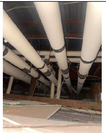
P2 – Straight runs fiberglass insulation
