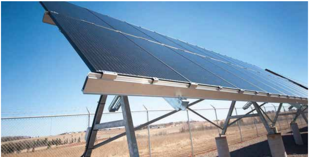
City of Summerside, announced funding to build a solar energy farm and storage facility in Summerside. The project involves the construction of a new 21-megawatt solar farm and a battery storage facility.
