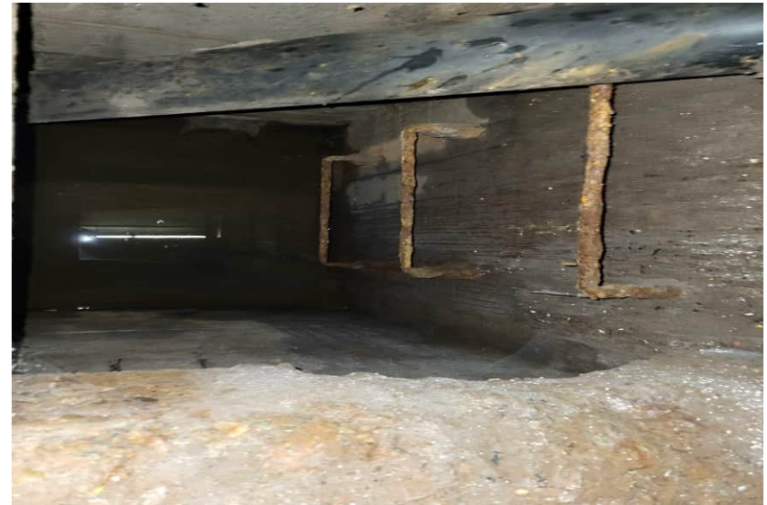
8. Interior oil water separator collection pit.
