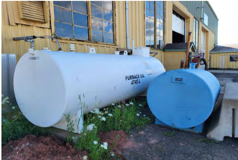
9. Two ASTs located adjacent to the northeast side of the government garage.
