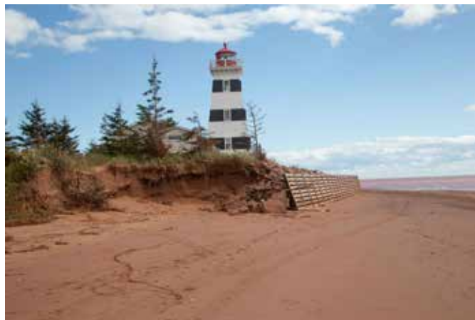
Figure 33. End-scouring on Langley Sea Wall at West Point (D. Jardine, 2019)
