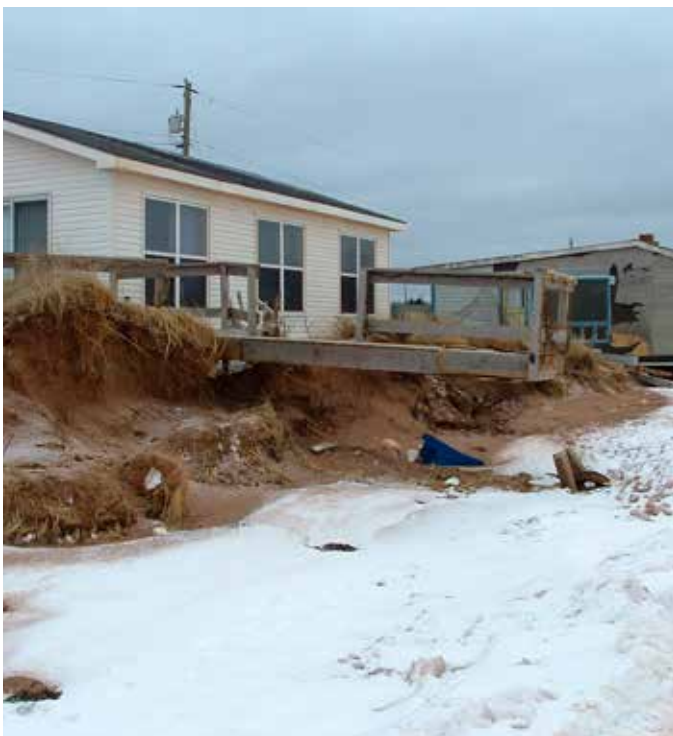
Figure 73. Waterfront cottages damaged in a severe storm event. Maximeville, Egmont Bay PE (D. Jardine, 2006)
