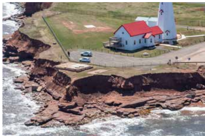
Figure 28. Coastal erosion at East Point where an old foundation is located at the top of the cliff (H. Parnham, 2023)
