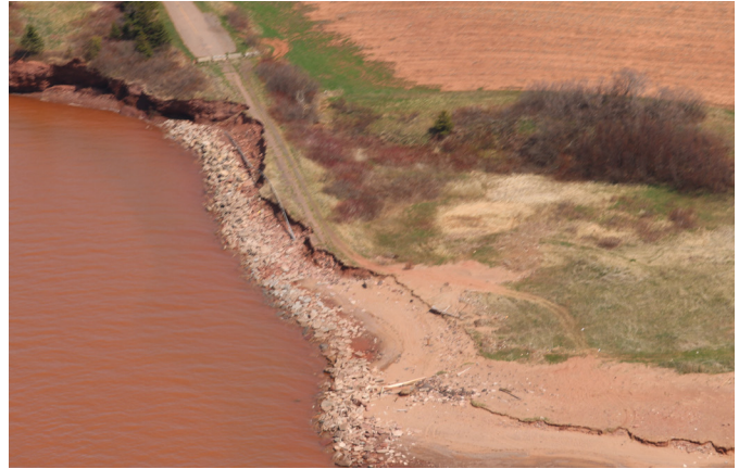
Figure 21. Brae Harbour road and wharf were abandoned rather than decommissioned. The beach at Brae Harbour road and is littered with the debris of the old structure. Brae Harbour, PEI. (H. Parnham, 2023)
