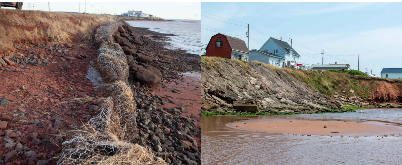
Figure 2. (left) Remnants of a failed gabion basket coastline installation. Victoria, PEI. (D. Jardine, 2015)
