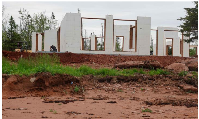
Figure 15. New construction of this summer home started with infilling the property to raise the foundation 3 m above high tide. Chelton, PE (D. Jardine, 2023)
